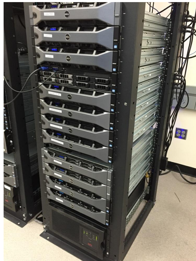
Our prototype system housed in FIU-SCIS data center
