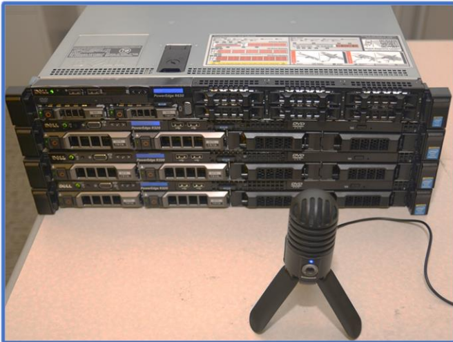
Dell PowerEdge servers
